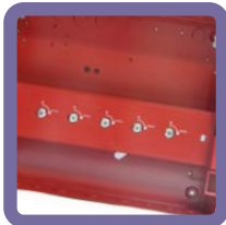
Disablement Switch Enclosure
